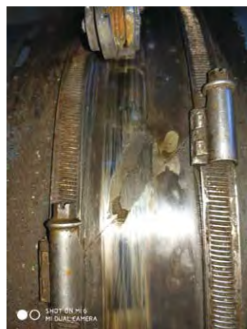
Slip ring in poor conditions
