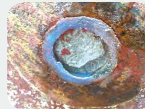
Ref. cell in poor condition
