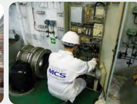
Fault finding on the ICCP power unit
