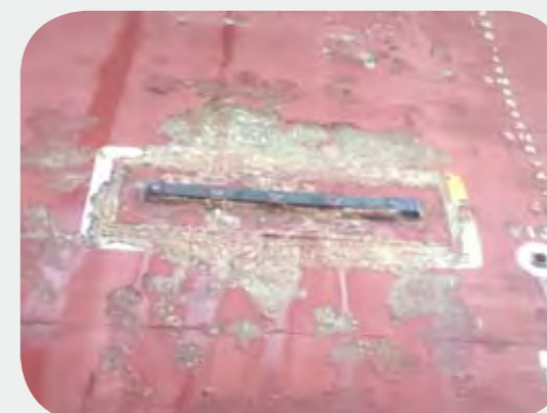
Di-electric shield in poor conditions
