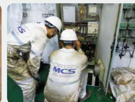
ICCP system inspections on the control panel
