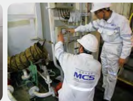
Inspection on mV meter for shaft grounding assembly
